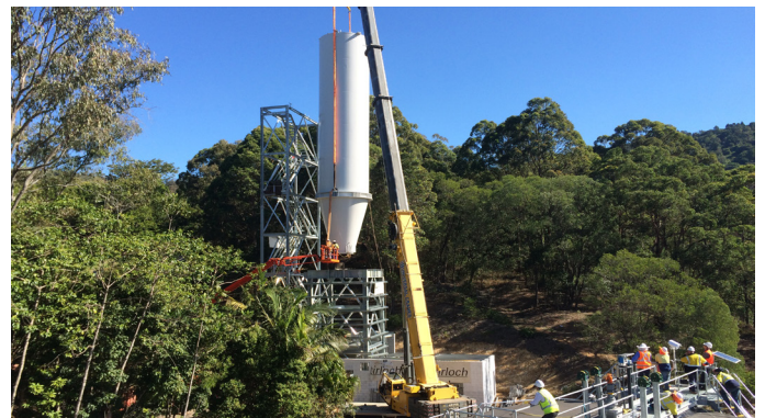
A new lime silo was installed in June 2016 and commissioned in March 2017 to improve the plant's capacity to cope with water quality challenges during heavy rainfall.
