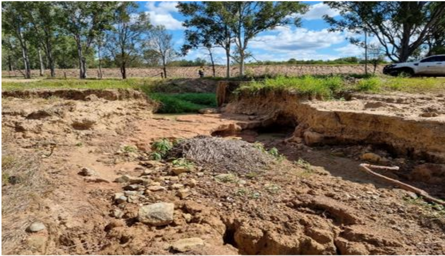
Figure 4: Washout damage on Brightview Channel
