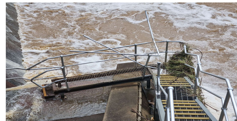
Figure 4: Cedar Pocket Dam damage to handrails
