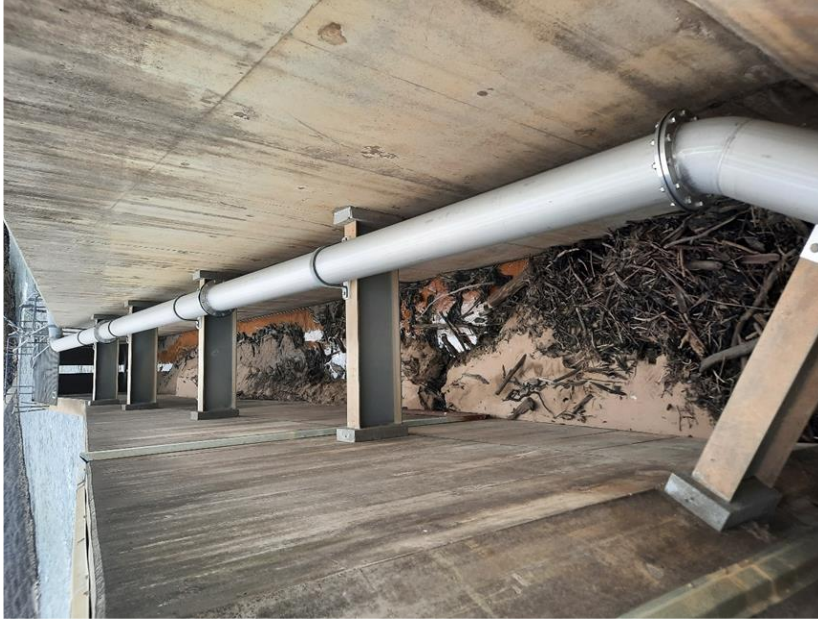
Figure 6: Cedar Grove Weir (Flood Debris in Fish Lock)
