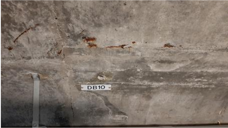
Figure 3: Maroon Dam conduit concrete spalling
