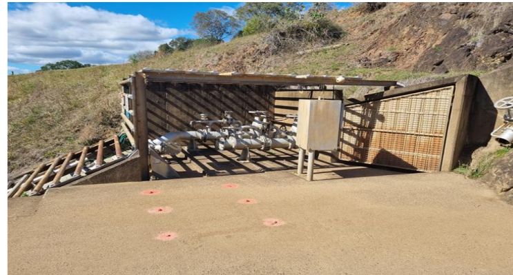
Figure 7: Pie Creek pump back to normal operation.
