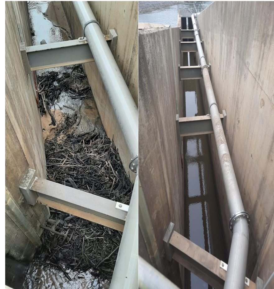
Figure 3: Cedar Grove Fish Loch Flood Debris before and after clean.
