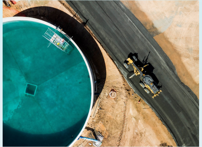
South West Pipeline Wyaralong Transfer Station
