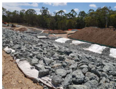
rock lined drains are being installed. During heavy rain events, these drains will move water away from the dam wall.
