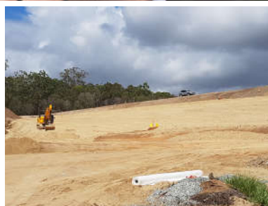
the beach! This is the Leslie Harrison Dam wall with new sand filter layers being installed.
