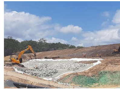
Massive drains will carry water around the dam wall to protect it from erosion.
